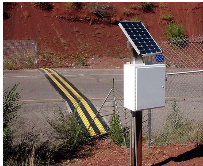
Electro-mat, Electrobraided fencing, 8-foot fence and solar collector on N.M. 333.
